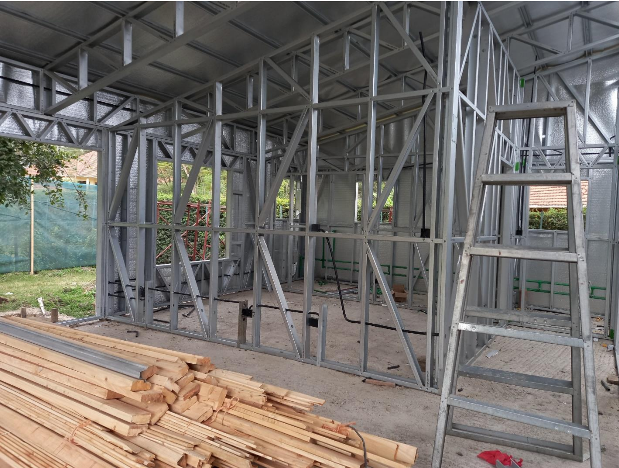
Photo 07: Light gauge steel and Mild steel sections framing with timber in-fills on concrete floor surface.
