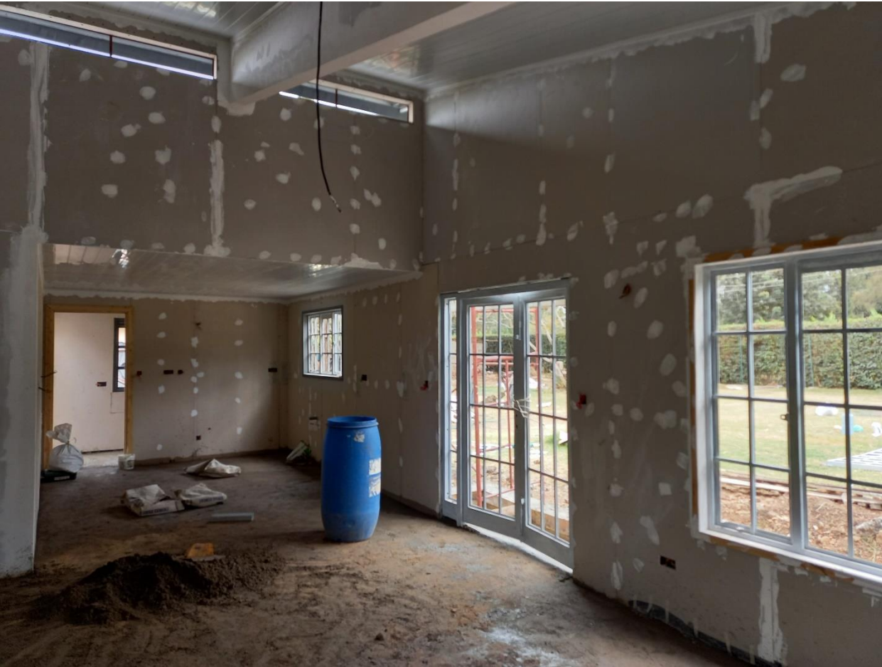
Photo 09: MDF cladding internally and Gypsum boards for the ceiling; painted to approved colours..
