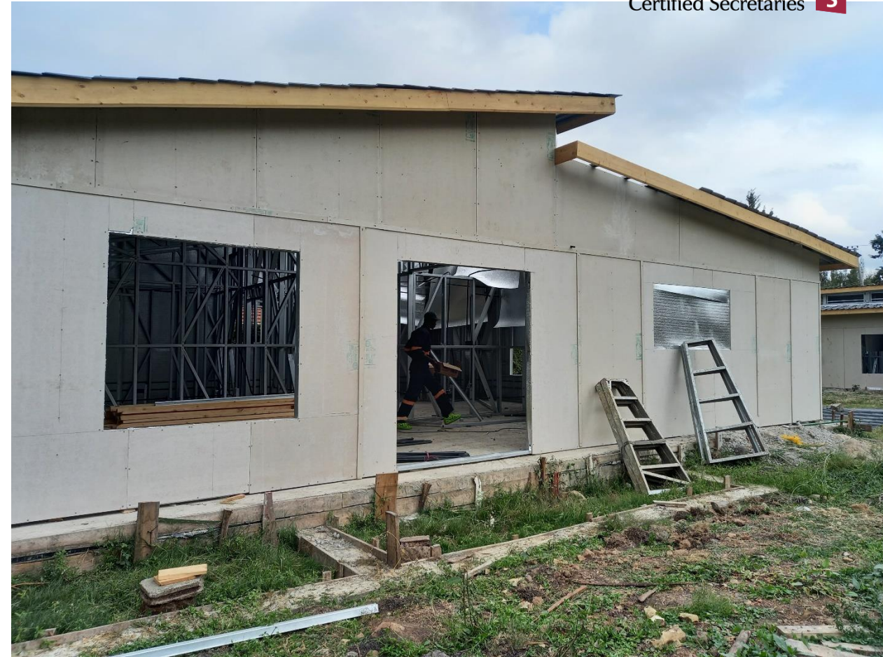
Photo 08: Waterproof MDF panels on external cladding finished with Rough and Tough all weather paint.
